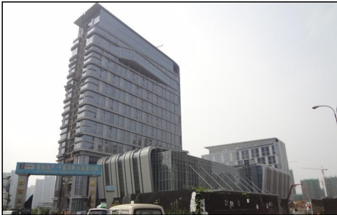
Crowne Plaza Chengdu Wenjiang and Holiday Inn Express Chengdu Wenjiang Hotspring hotels under construction
